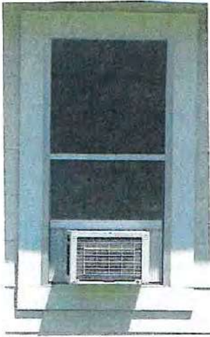
When adding modern amenities, their installation should avoid irreparable physical or aesthetic damage to the residence.
