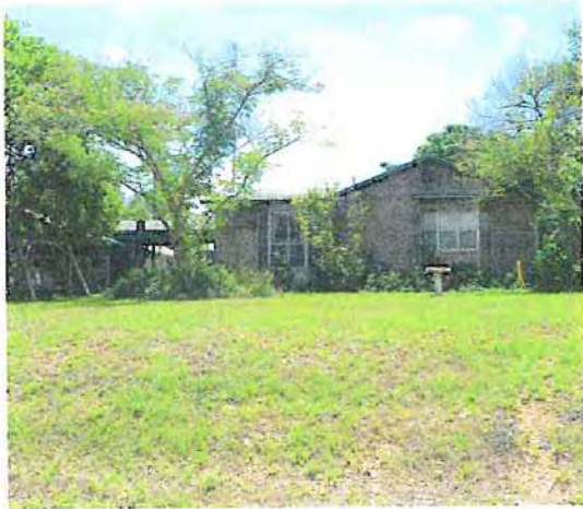
The material of the window helps to date the construction. Retaining the original window material is important to preserve that character.
