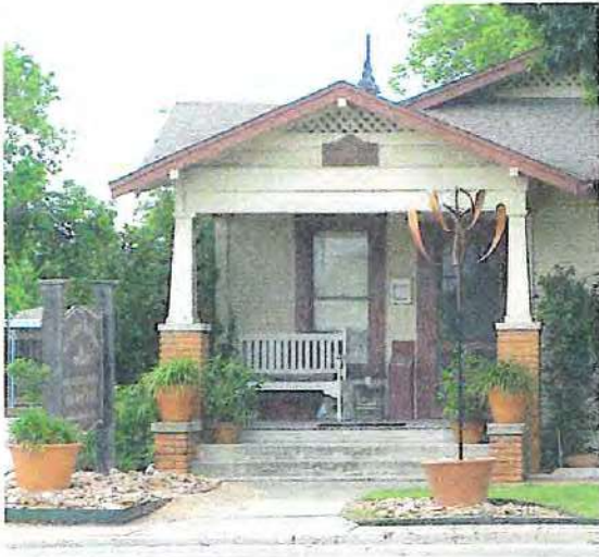
Brick detailing should be retained as it is a contributing factor to the character of a building.
