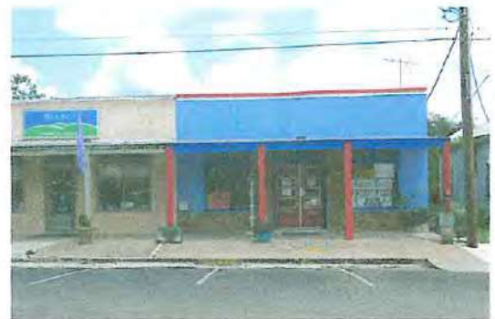
Stucco should not be added over historic building materials as it damages the historic materials and changes the scale and profile of the original.
