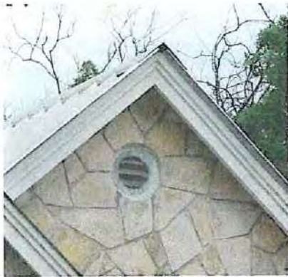
A wooden louver vent.
