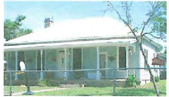
The type of roof form plays an important role in defining the character of the residence.
