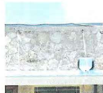
A through-wall scupper and conductor head.
