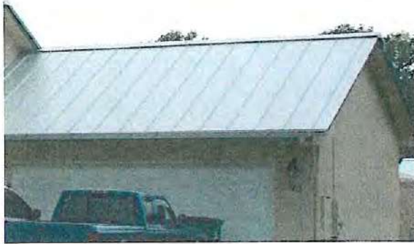
This contemporary standing seam metal roof is installed with a ridge cap, gutters, and downspouts.
