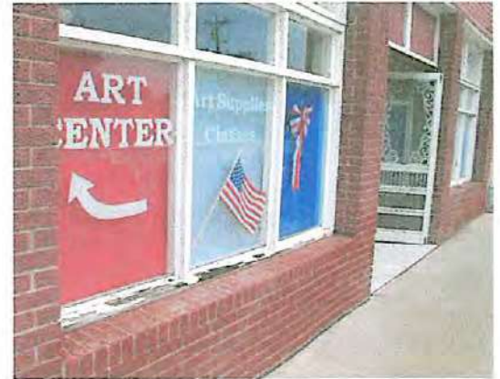
When necessary, replace missing or badly deteriorated wood.
