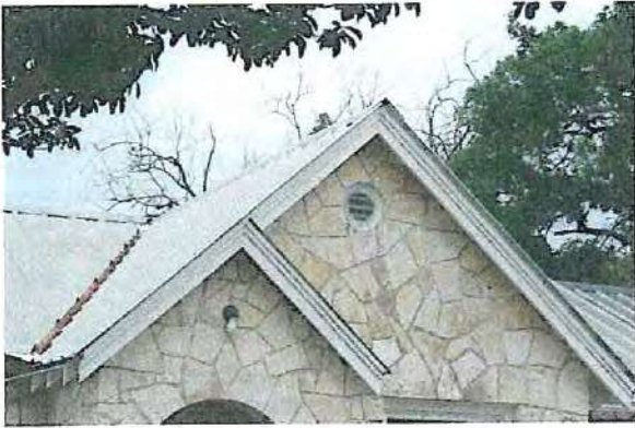
Maintaining the roofing material and flashing is crucial to the longevity of a roof.
