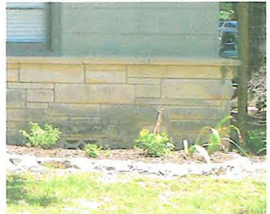
An under-floor vent in a masonry skirt .
