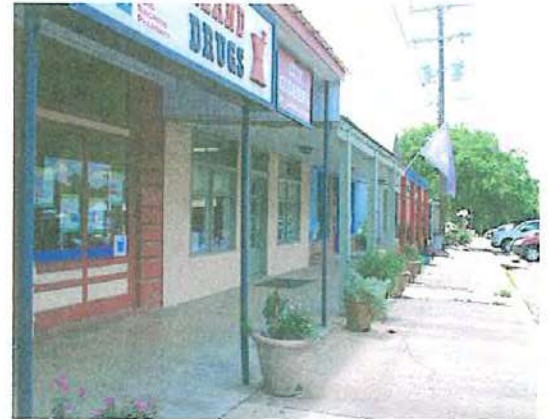
Canopies along with their attachments, anchors, and structure should be regularly inspected.
