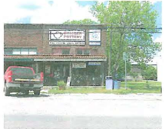
Boarded-up openings should be restored.
