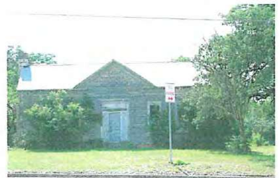
Addressing issues that will prolong the life of the building should be attended to first.
