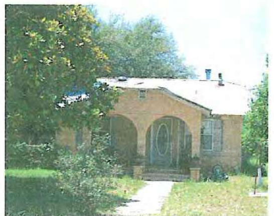
When replacement windows are not consistent with the original material and/or proportion, consideration should be given to replacing them to match the original.
