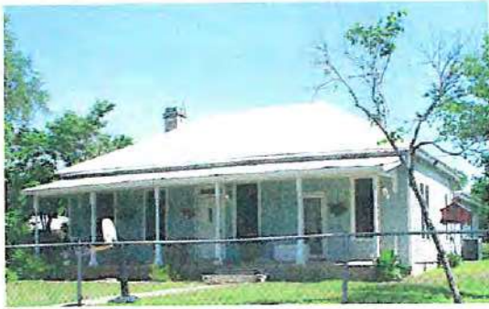
Regular maintenance to porches is necessary due to their exposure to the elements.
