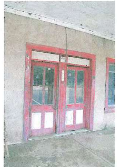
Wood and metal building components should be maintained with paint to protect it from deterioration.
