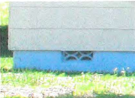
Vents along the perimeter provide necessary ventilation under the house.
